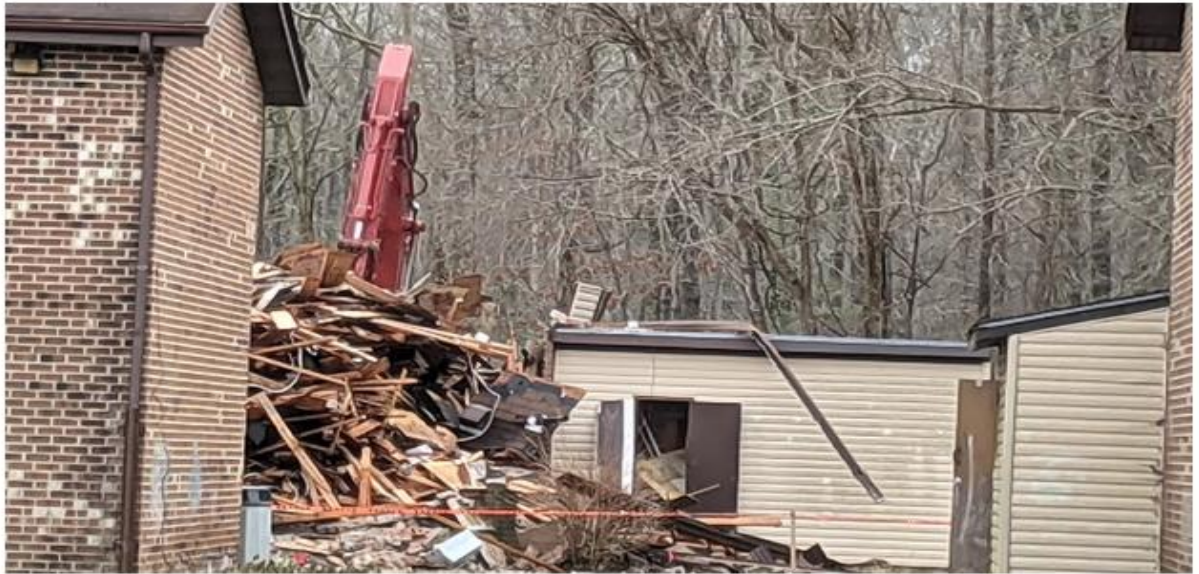
Demolition of the old Parker Riddick apartments was under way this week.
